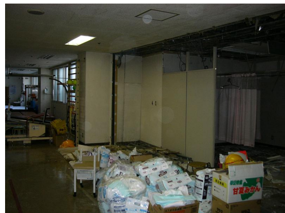
Photo 4. Damage to ceiling, Ojiya Hospital.
