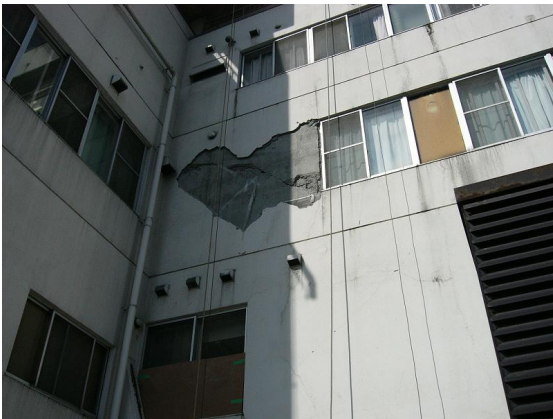
Photo 1. Exterior wall peeled off, Ojiya Hospital.
