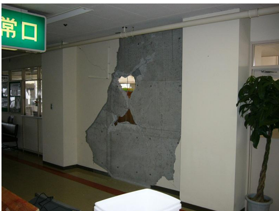
Photo 3. Interior wall peeled off, Ojiya Hospital.
