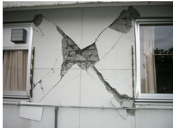
Photo 2. Exposure of reinforcement, Ojiya Hospital.
